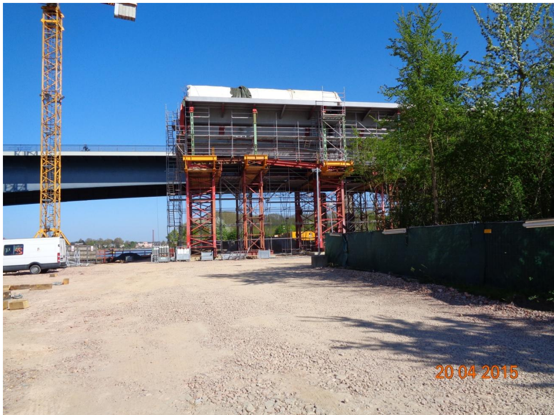
Fig. 40 Construction of bridge with the supporting structure and the auxiliary foundations, middle part of the Schierstein bridge
