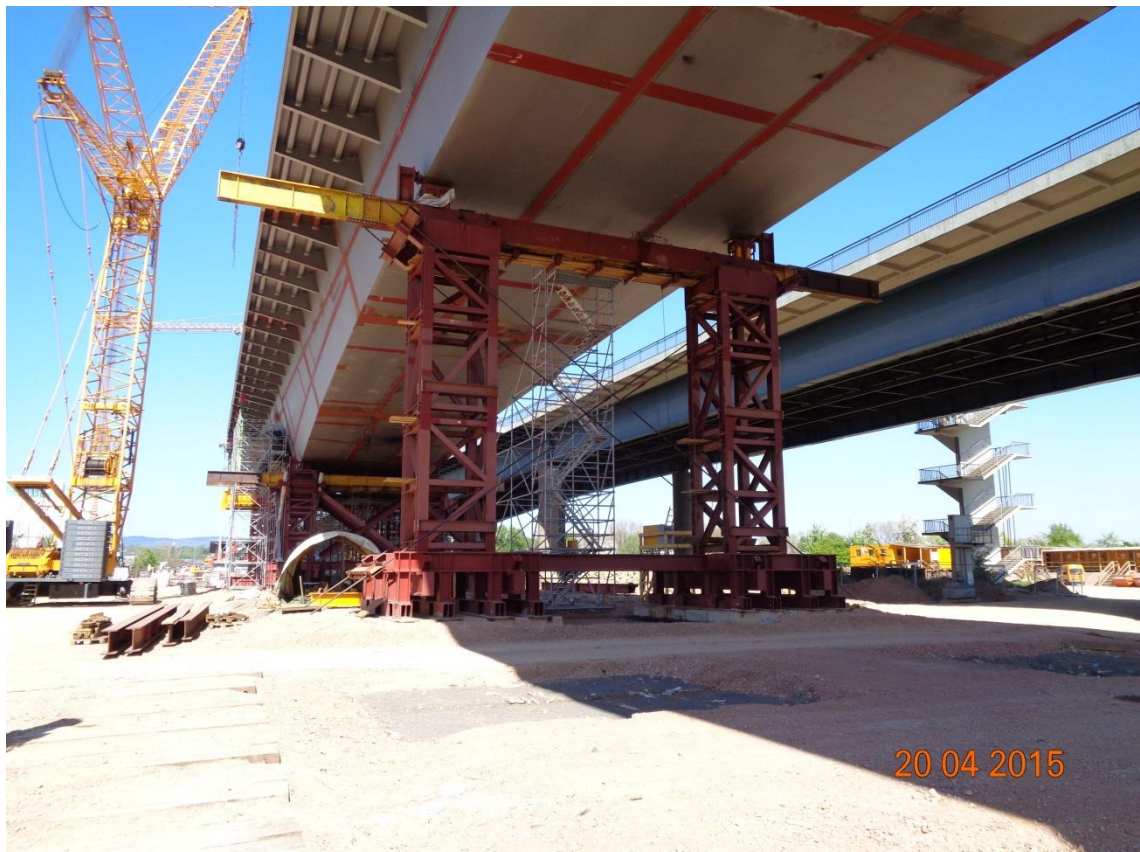
Fig. 1 Bridge construction with the auxiliary foundations, Schierstein Bridge between Mainz and Wiesbaden, Germany
