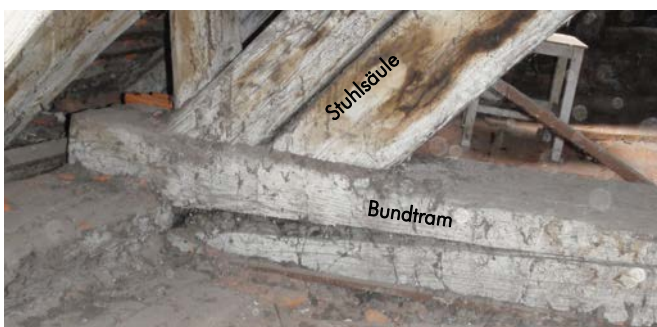
Bild 13. Querzugversagen des Bundtrams. Fig. 13. Failure of tiebeam due to stresses perpendicular to grain.
