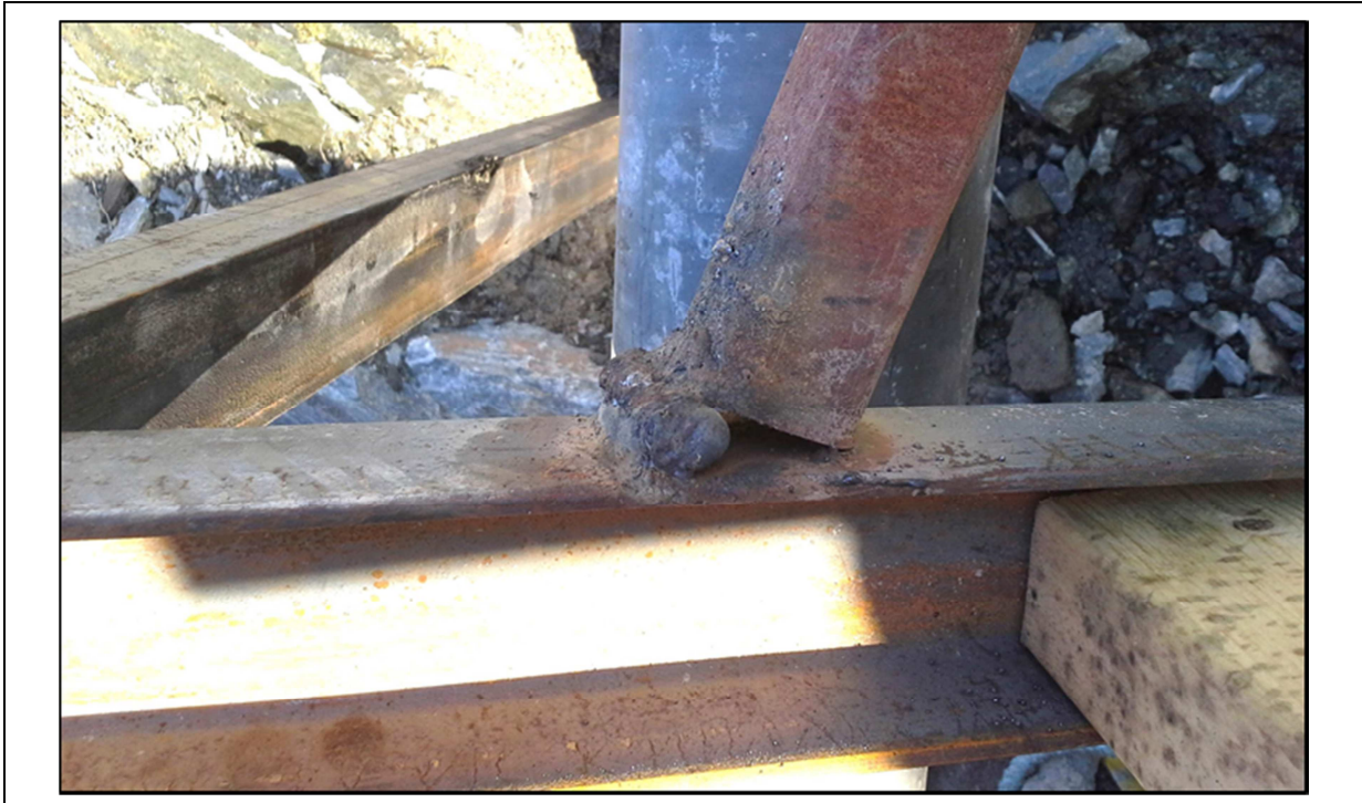
Figure 5: Poor execution of a weld joint
