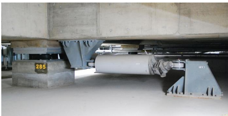
Figure 6.36 Installed Oil Damper. 246
