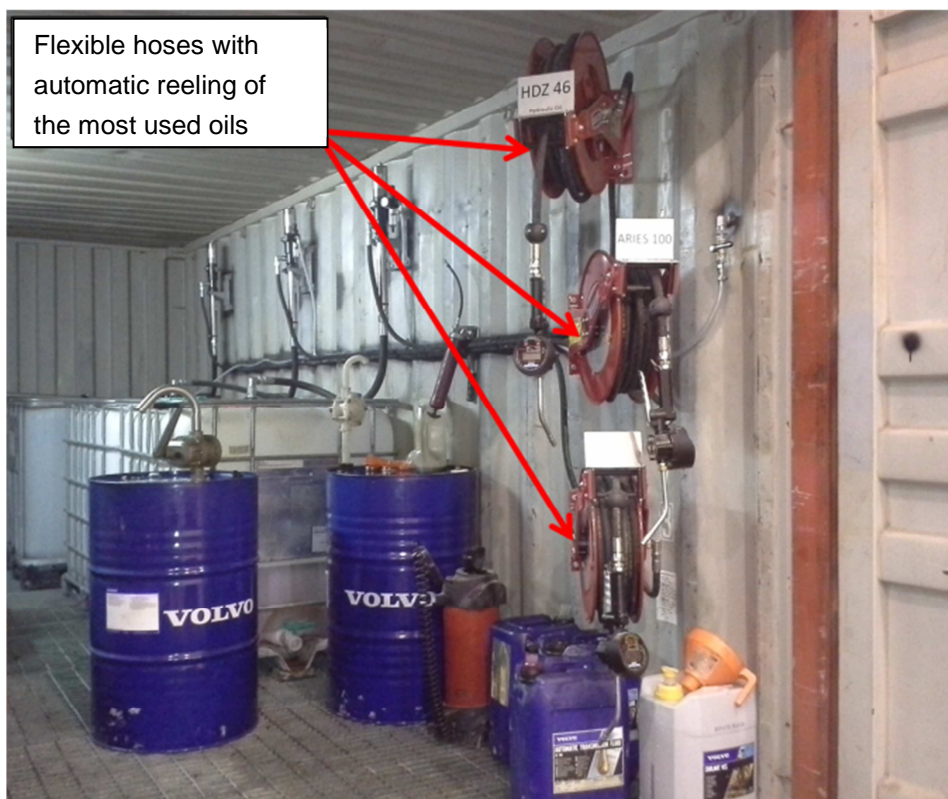
Figure 38: Central oil distribution at the machine workshop
