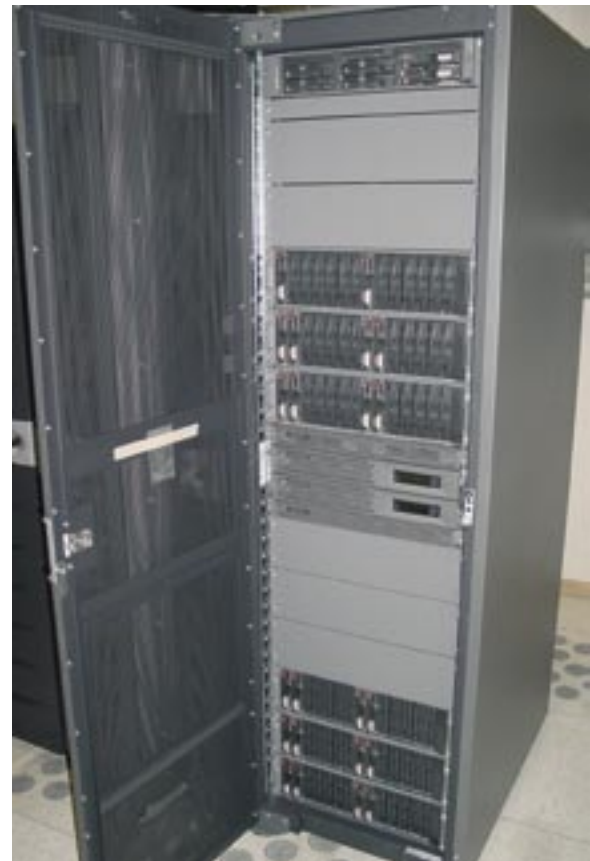
SAN (HP EVA, 1.5 Tera Byte, Fibre Channel Technology)
