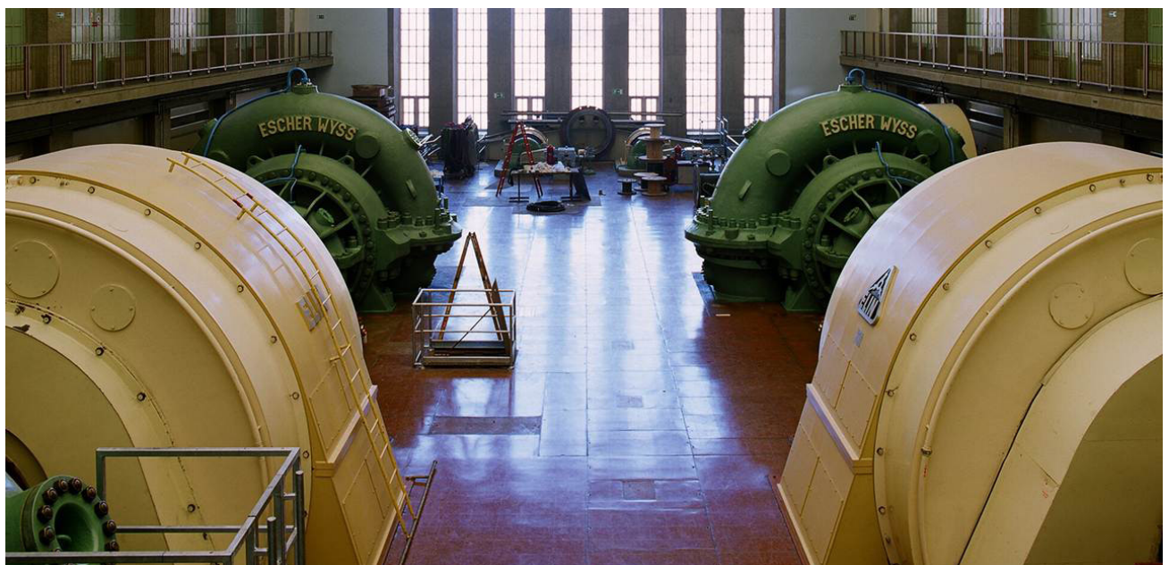
The power house with ternary machine units of Limberg I [ 5 ]
