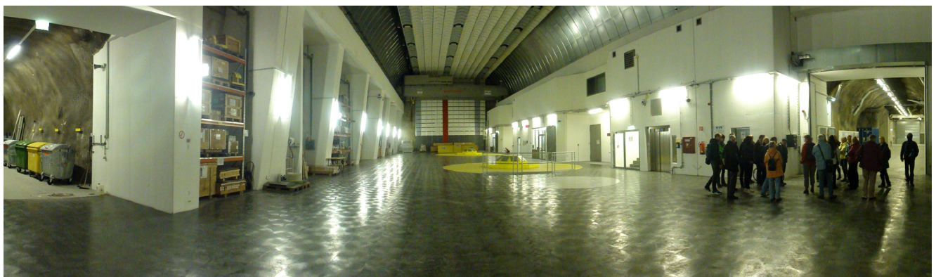
View at the machine hall of Limberg II [ 11 ]
