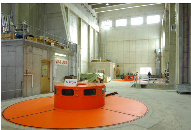
Machine hall in the power house Feldsee in 2011 [ 1 ]
