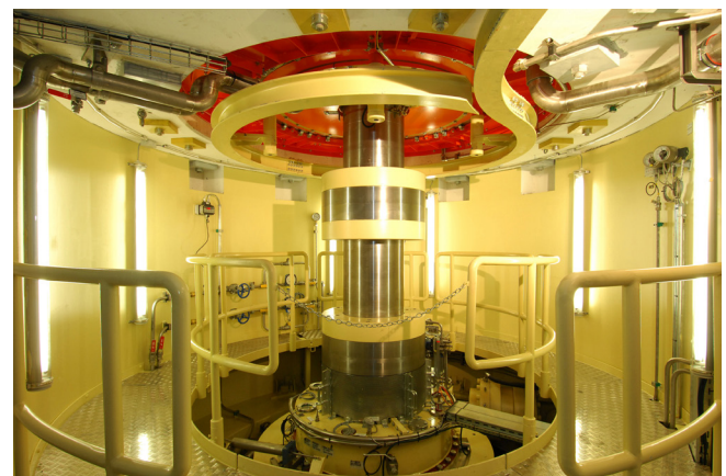
Shaft between the reversible pump turbine and the motor-generator in 2011 [ 1 ]
