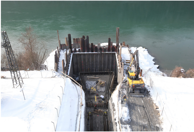
Inlet structure at the river Drava [ 4 ]
