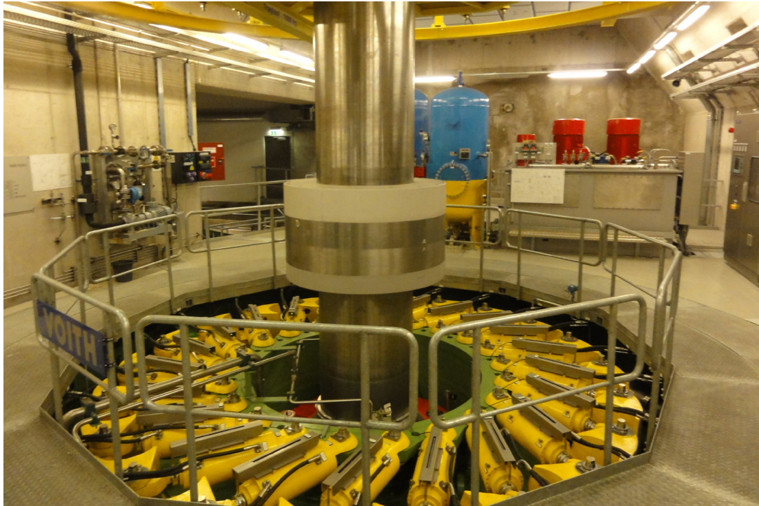
Generator room of Limberg II [ 4 ]
