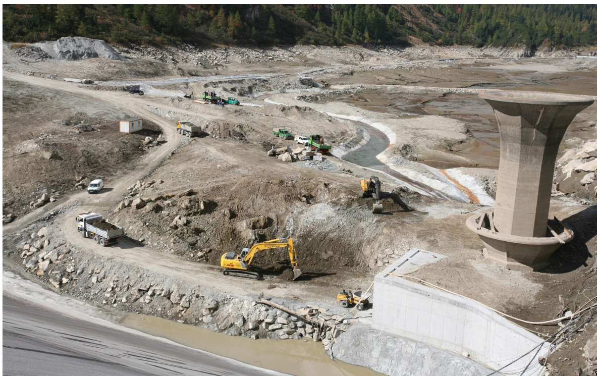
Construction site at the reservoir Wurten with the inlet/outlet and the spillway in shape of a trump in 2007 [ 1 ]
